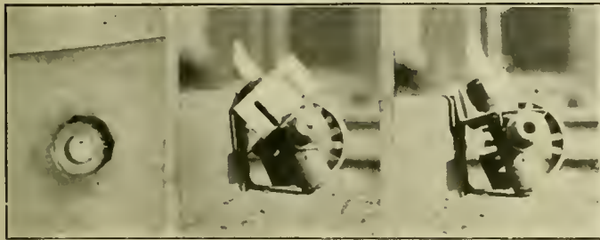
Fig. 2—Showing Opening in Boiler, Gauge Cock Opening Showing Scale and Same Opening with Scale Removed
